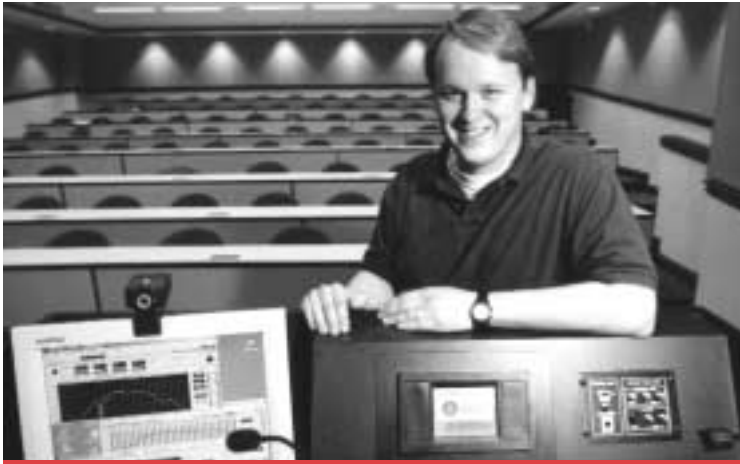
Classroom audiovisual technology in the Dedman Life Sciences Building is controlled from a podium workstation designed and installed by NCMIT staff. David Alley, NCMIT technology support manager, inspects the workstation in the Harold Jeskey Lecture Hall.
